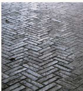
2005年紅樓荷造場紅磚地坪 黃俊銘研究室提供 Brick pavement within the packaging Area of the Red House, 2005 Provided by Huang Chun-ming Architectural Research Lab
